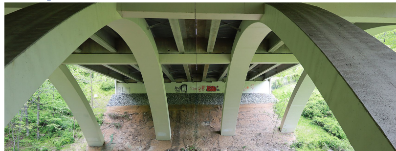
Image: MD 200 crossing Rock Creek, wide arch facilitates wildlife crossing credit: wikiwand.com
