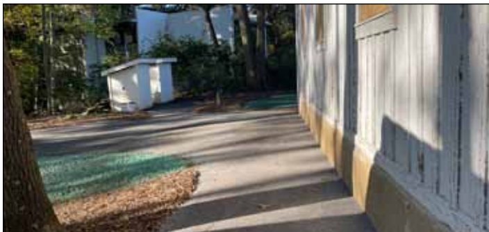
Trail work on the southeast side of the School by Alex's ProScape.
