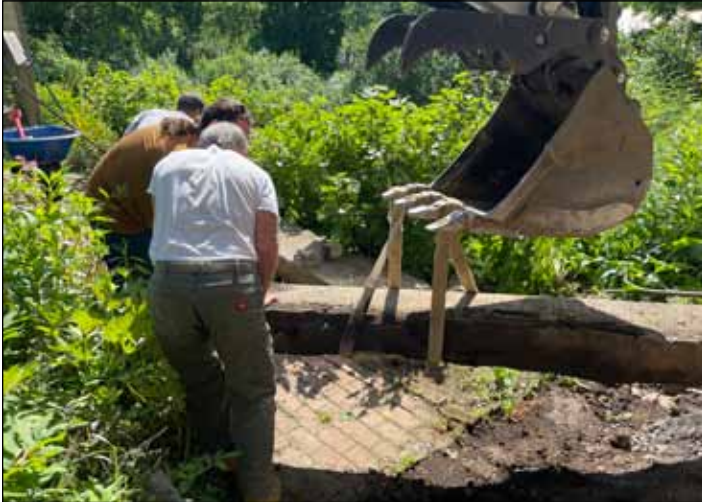
Alex's ProScape assisting Philip Hawk with their equipment to reset the stone steps from the porch to walkway.
