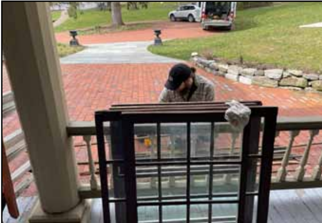
Haven Tucker with Anders Olsen Construction and Renovations preparing to re-install restored window sashes.
