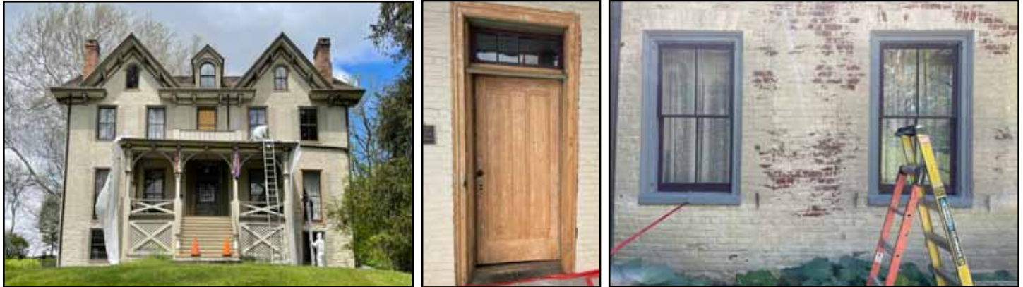
Left to right: Work on the south-front elevation of the Mansion, west porch door into the period kitchen after the paint had been removed from the door and door frame, preparation of the brick before priming and painting.
