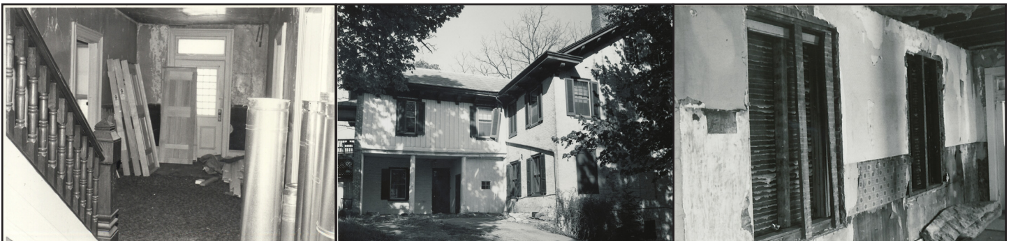
The Centre Furnace Mansion 1979-1983 prior to restoration. Left to right: First floor main hall after wood paneling had been removed, rear ell with portion of porch enclosed, 2nd floor (current library) showing where 2nd floor porch windows had been enclosed.
